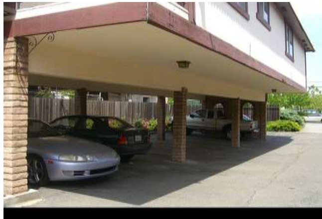
Fig 1.1 Example of a soft storey at the ground floor
